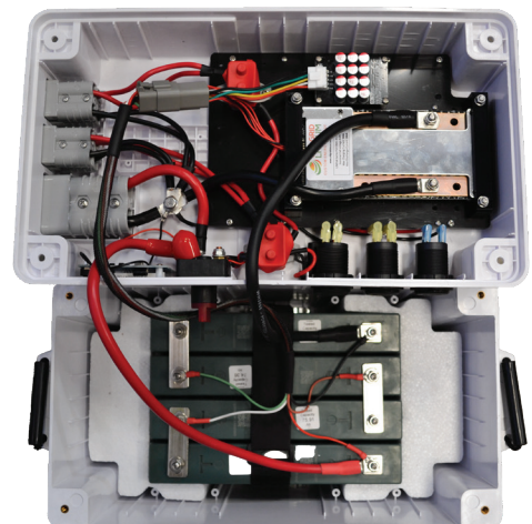
OGL BATTERY BOX
